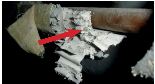
Asbestos corrugated paper as insulation.
